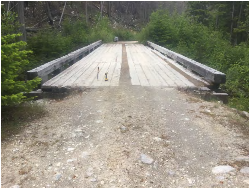
Loosing fill on road approach to right abutment
